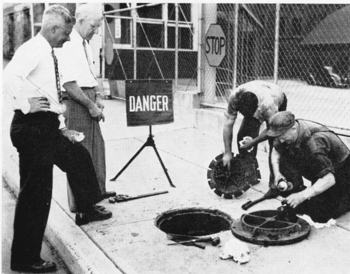
Time for a check-up. Mr. M. A. Cummings, Factory Mutual Engineer, was on hand last week for his periodic inspection of double check valves in the Main Plant.
